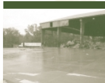
The brutal winter weather forced OCRRA to replace the unloading deck area.
